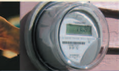
Automated Meter Reading
